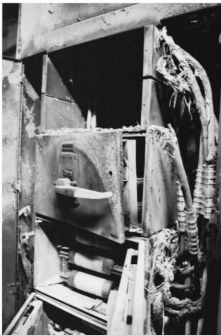
Figure III – This power switchboard burn-down probably started as an arching ground fault and escalated to a phase-to-phase fault before the main circuit protective device opened. It is testimony to the destructive force of “available short circuit current” that can be supplied by your serving utility, and why the National Electrical Code says that your electrical system must be capable of handling it.
