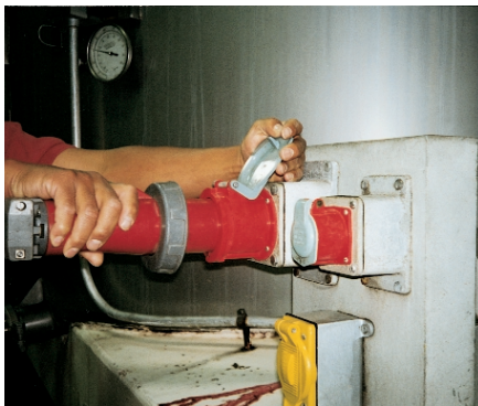
Figure I – Since this receptacle provides a means to disconnect a portable pump from its source of electrical power, it is by definition a “disconnecting device.” The National Electrical Code states that any such device in a motor circuit must be “horsepower rated.” This pin-and-sleeve device is not.
